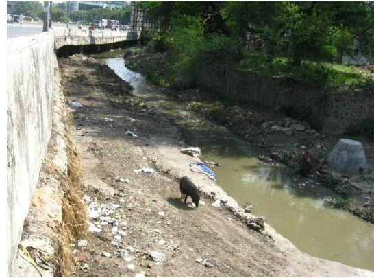
Photo 14: Condition of Channel at Bibvewadi
