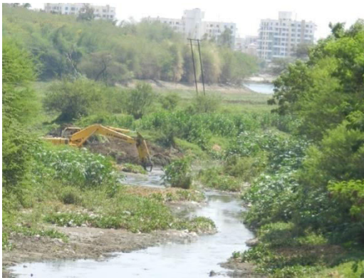
Photo 7: Sewage dumping in channel (Pashan Gaathan)
