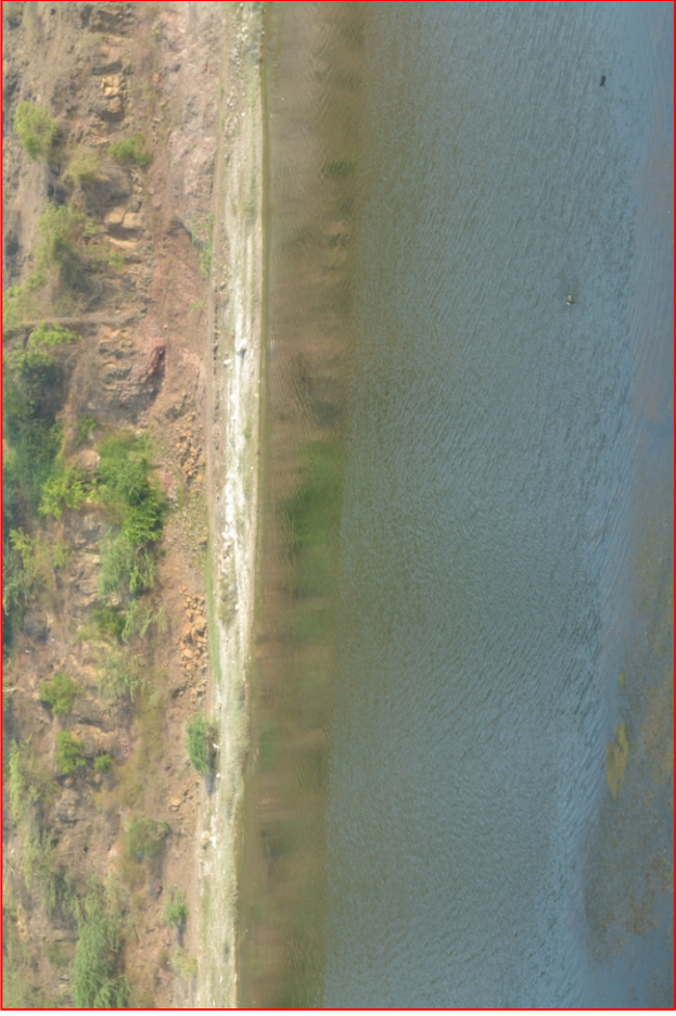
Narsingpur-Nira river erosion of river bank
