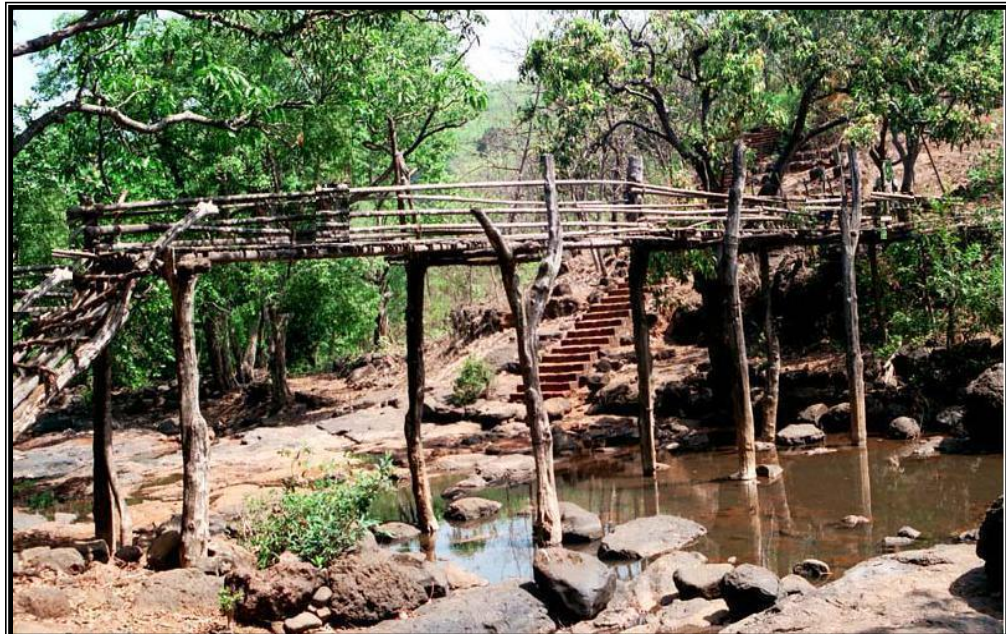
A Traditional Wooden Bridge on the way of Shri. Keshavraj Temple - Asud, Dapoli
