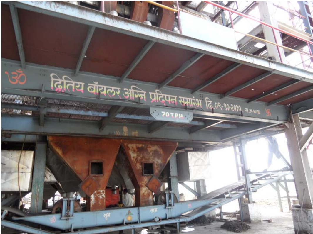
Boiler Section of NSAI.
