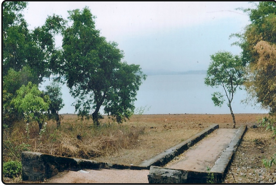
Bad Road of Vaitarna Dam
