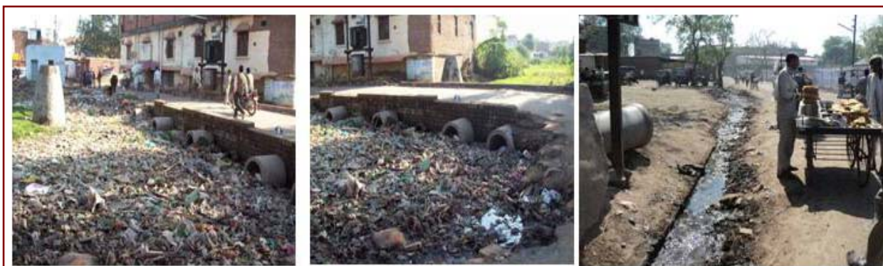
Photo: 4.1 Condition of open drains in the city
