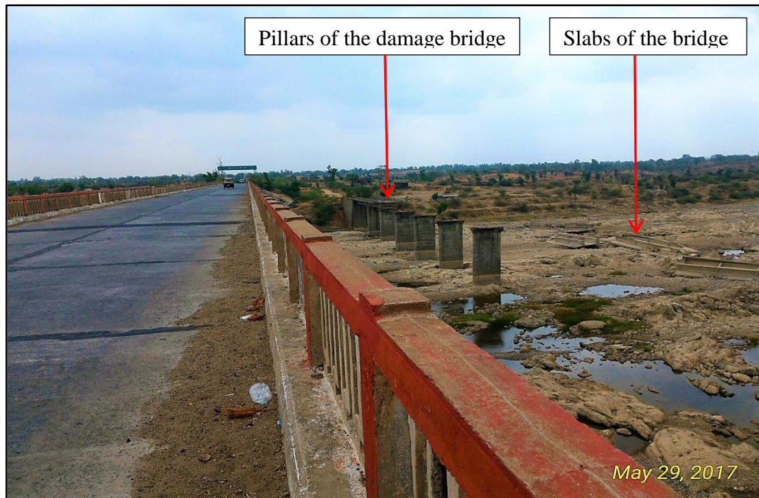
Figure 4.46: A view of collapsed Mahi Bridge by flood on 08/09/1973 from new bridge on the Banswara-Sagwara highway near Kailashpuri (Sagwara, Rajasthan)
