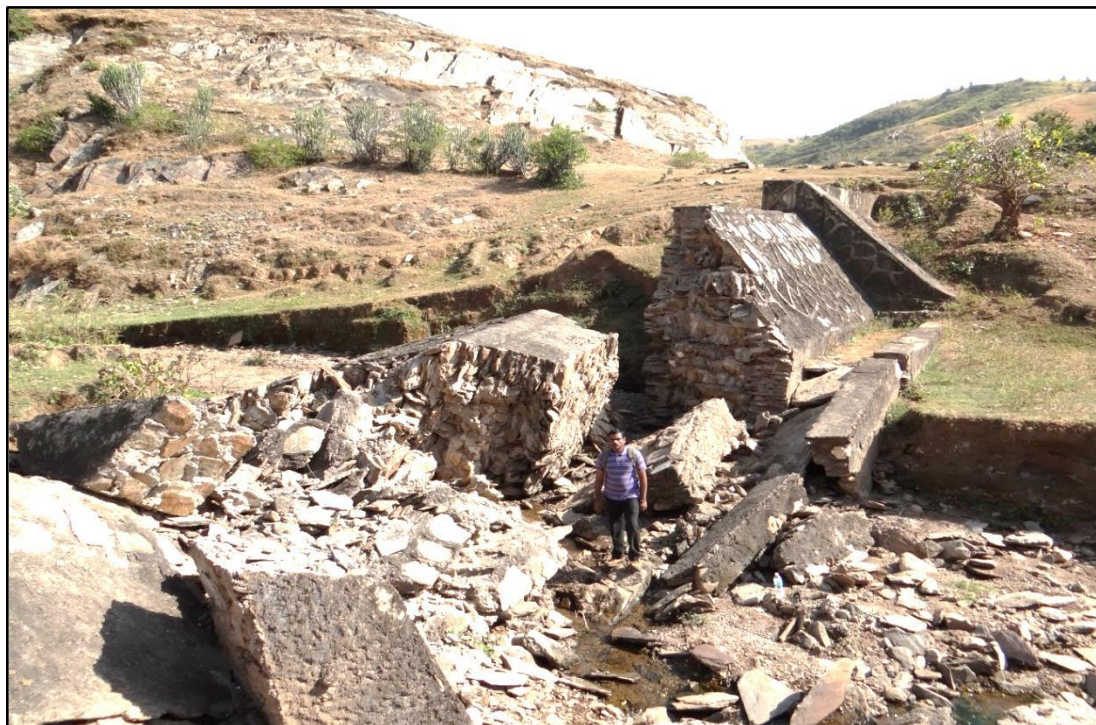
Figure 4.48: A weir on small stream of the Som River damage during 2006 flood at Saroli (Kherwara, Rajasthan)
