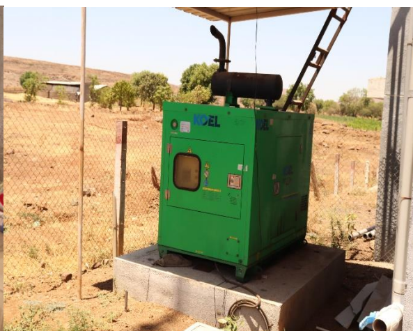
Image 76 – Generator in the backyard
