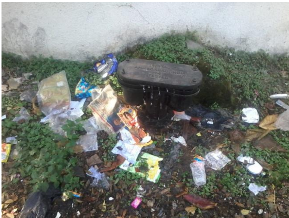
(d) Air valve of drinking water pipe line surrounded by solid waste material
