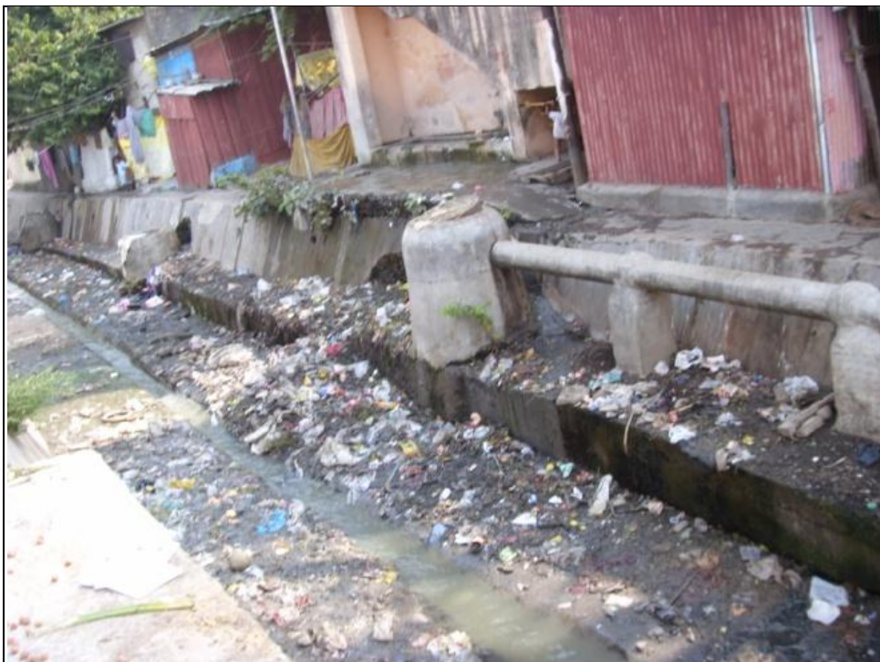
(b) Polluted dirty water drainage in Gawali Nagar slum
