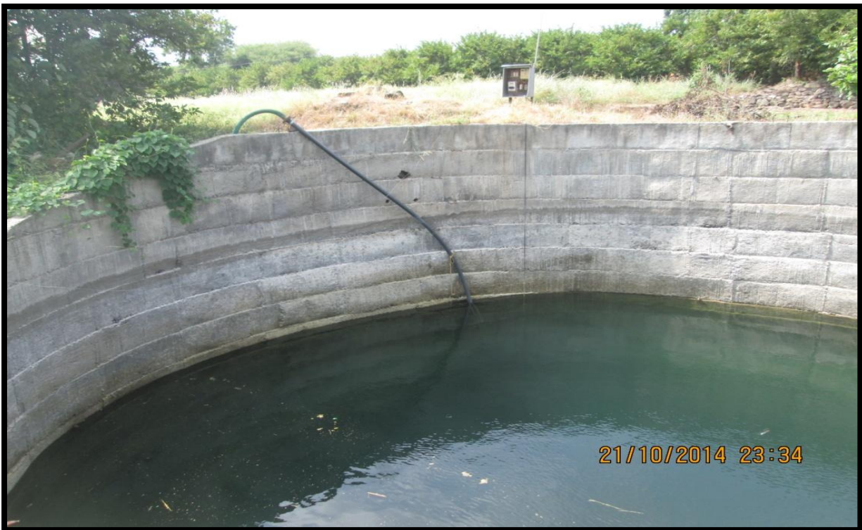
4. HIGH GROUNDWATER TABLE AT PIMPLE
